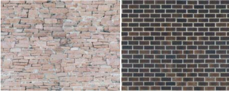
Reface of clay brick wall with KF-H by refilling of seams and coloration upon request.
