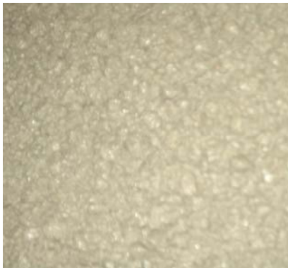
The texture and coloration of KF-F layer applied on a damaged concrete structure.
