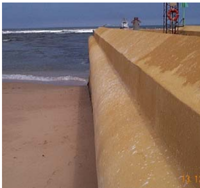
The rocky wall of light- house repaired by KF-SEA concrete and finished by KF-F prepared also with sea-water (Australia).
